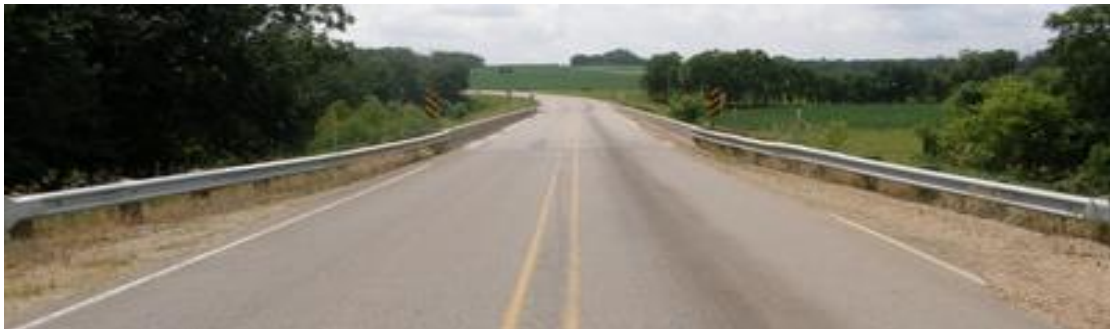
Figure 1: County Highway Bridge over the South Fork of the Iowa River in Hardin County, Iowa
